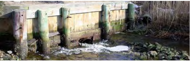
Under-sized culverts are barriers to the tidal flow and migration of fish. When natural tidal flow is restricted, the salt marsh ecosystems become degraded.
