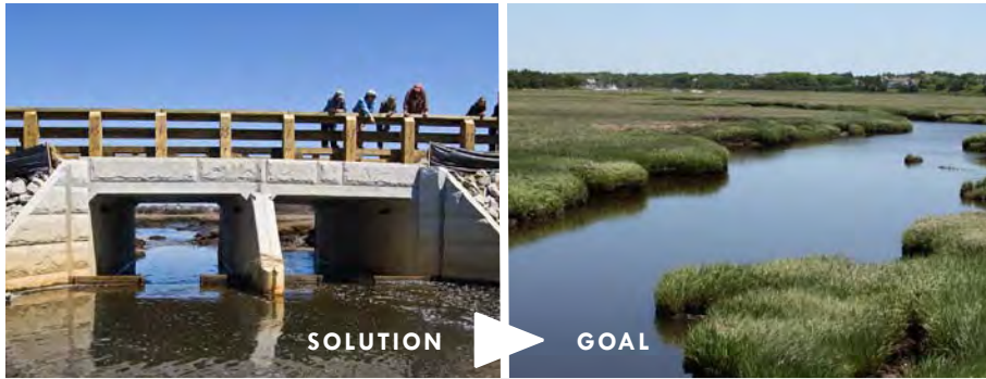
Installing larger culverts will restore normal tidal flow to salt marsh ecosystems.
